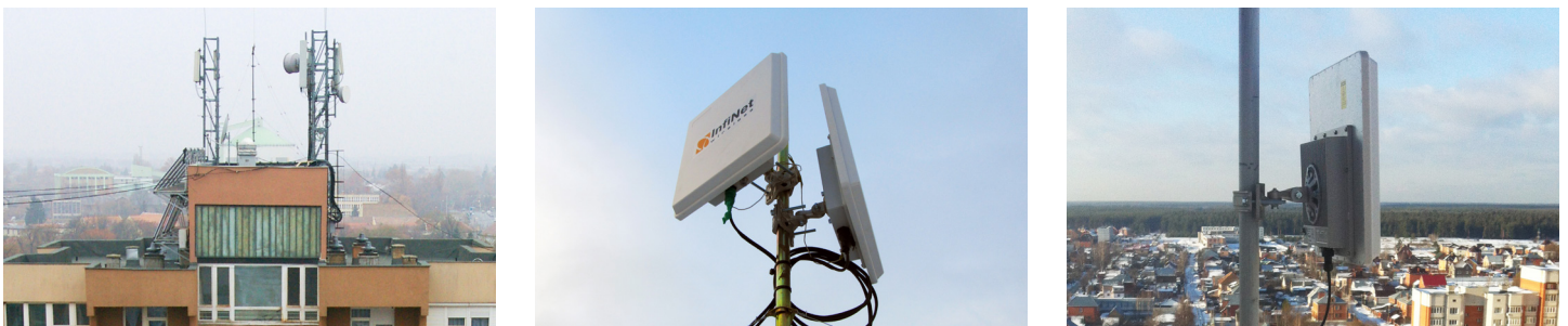
Figure 3 Street mounting of the InfiNet Wireless units
